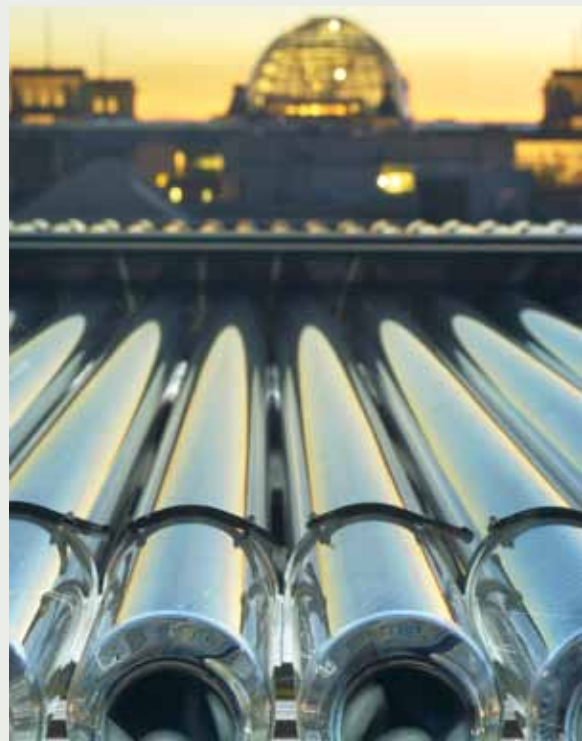
Thermal solar collection system on the roof of the Federal Government's Press and Information Centre Source: BSW-Solar/Langrock
